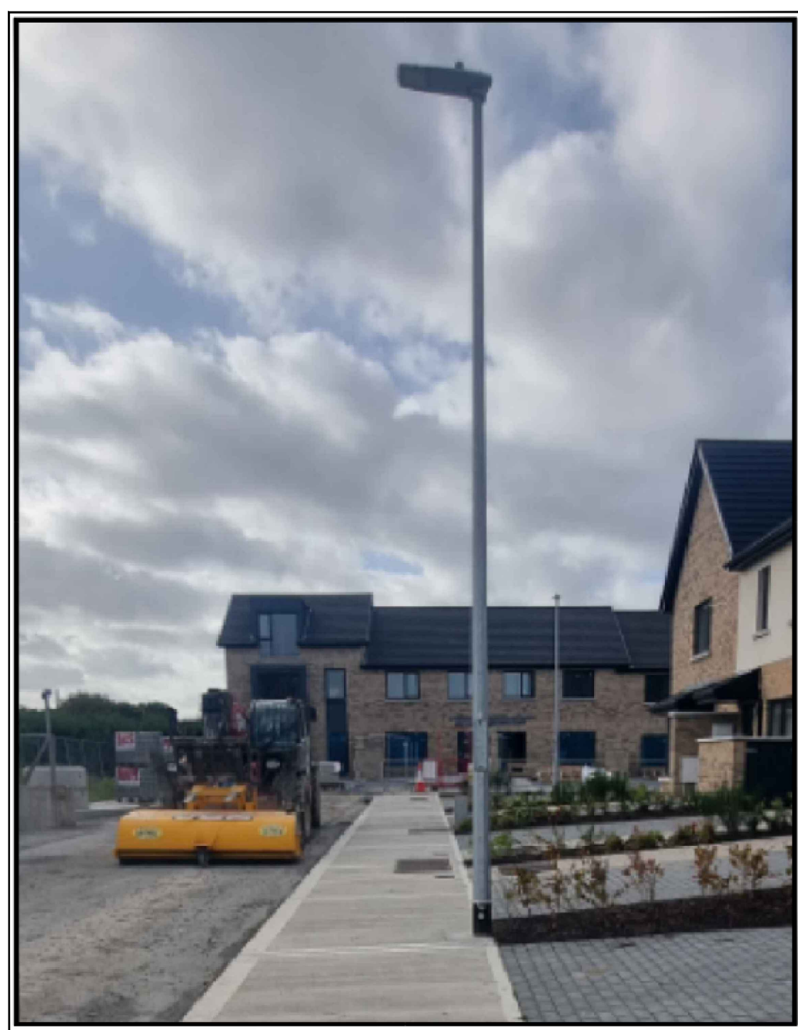
8M HIGH LIGHTING COLUMN TO THE REAR OF FOOT PATH OR ALONG ROAD PERIMETER
